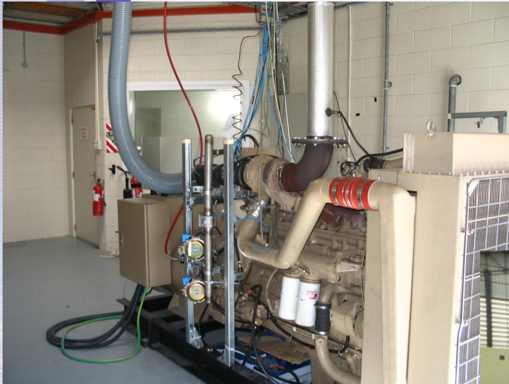
Dual Fuel Engines for Generators
