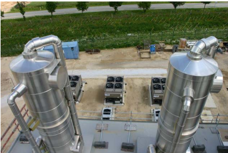
Greenlane® Biogas Upgrading Plant - Gustrow, Germany
