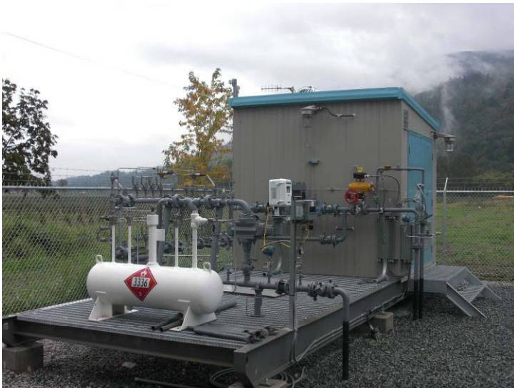
Terasen's Biomethane Measurement and Odourization Skid
