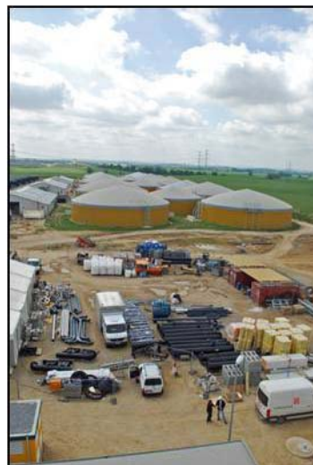
Anaerobic Digesters - Gustrow, Germany
