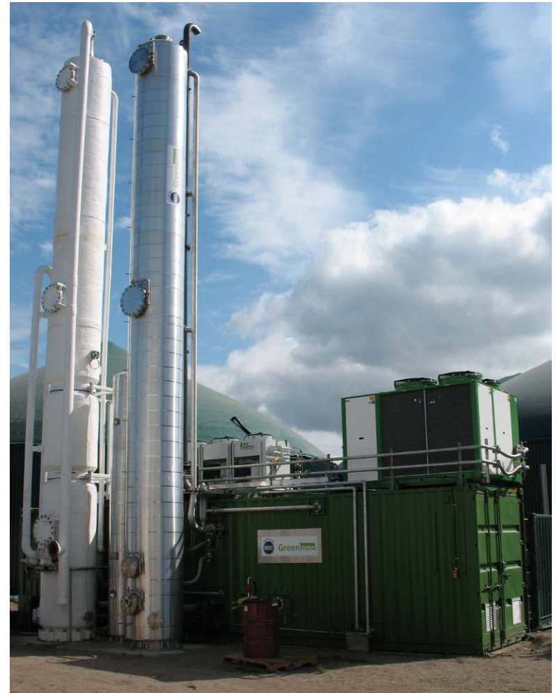
Catalyst Greenlane® RIMU – Fully Installed
