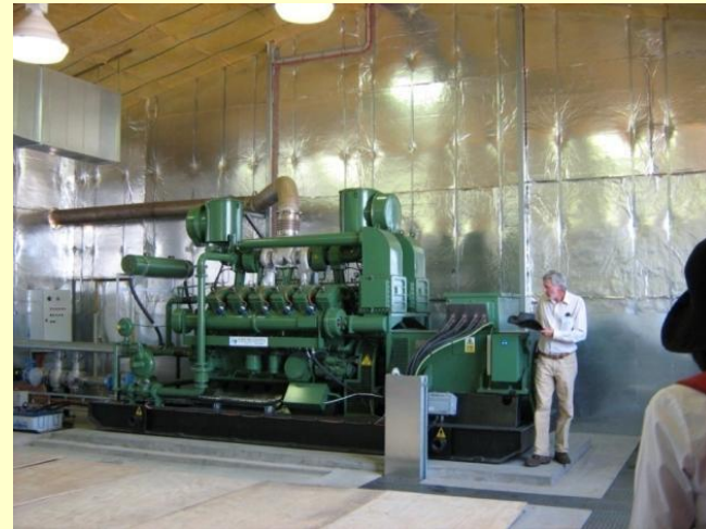
AJ Bush Digester and Gas Engine, Bromelton, Qld
