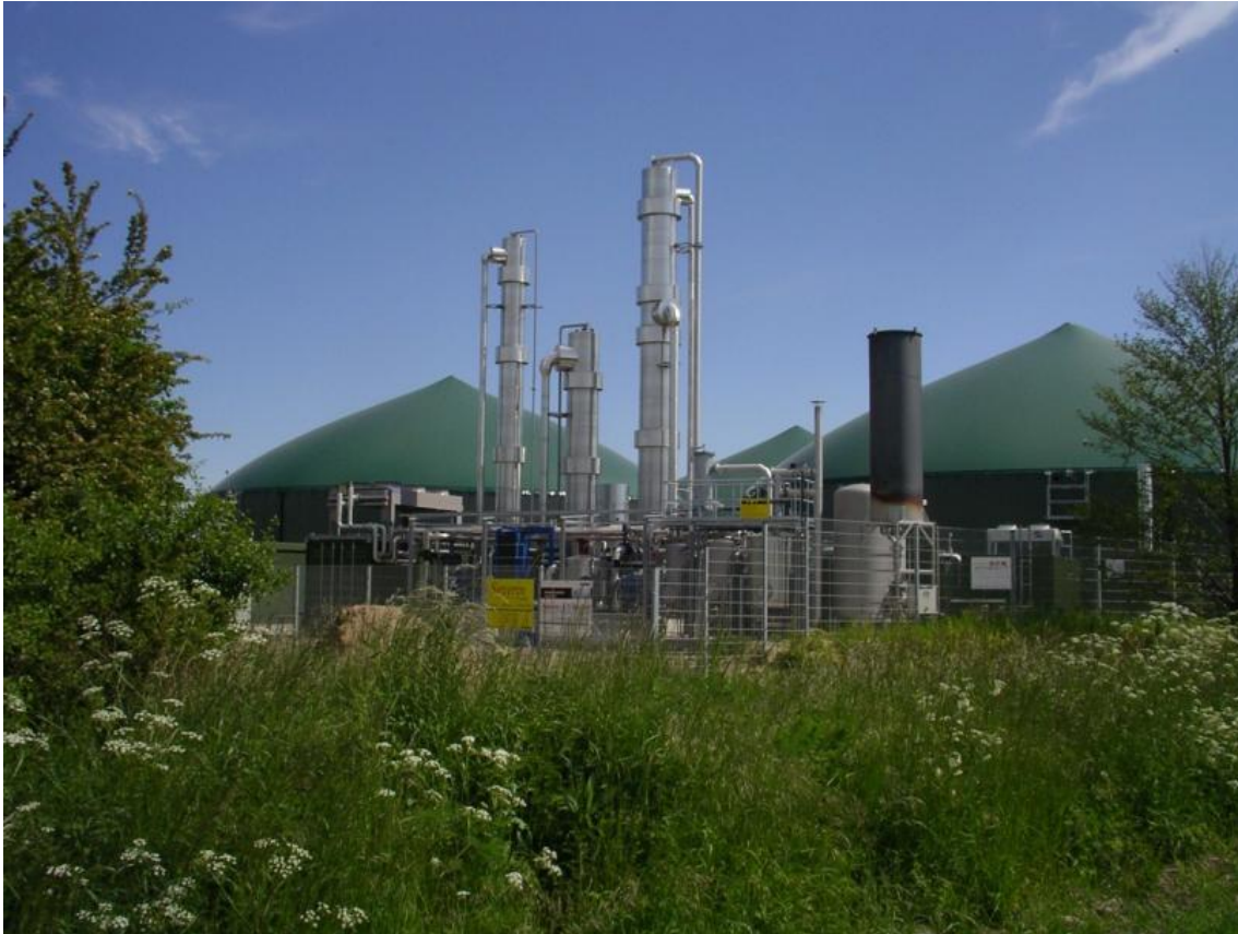
BIRO, near Hannover, Germany: 2.5 MW (thermal) biogas treatment for local grid connection
