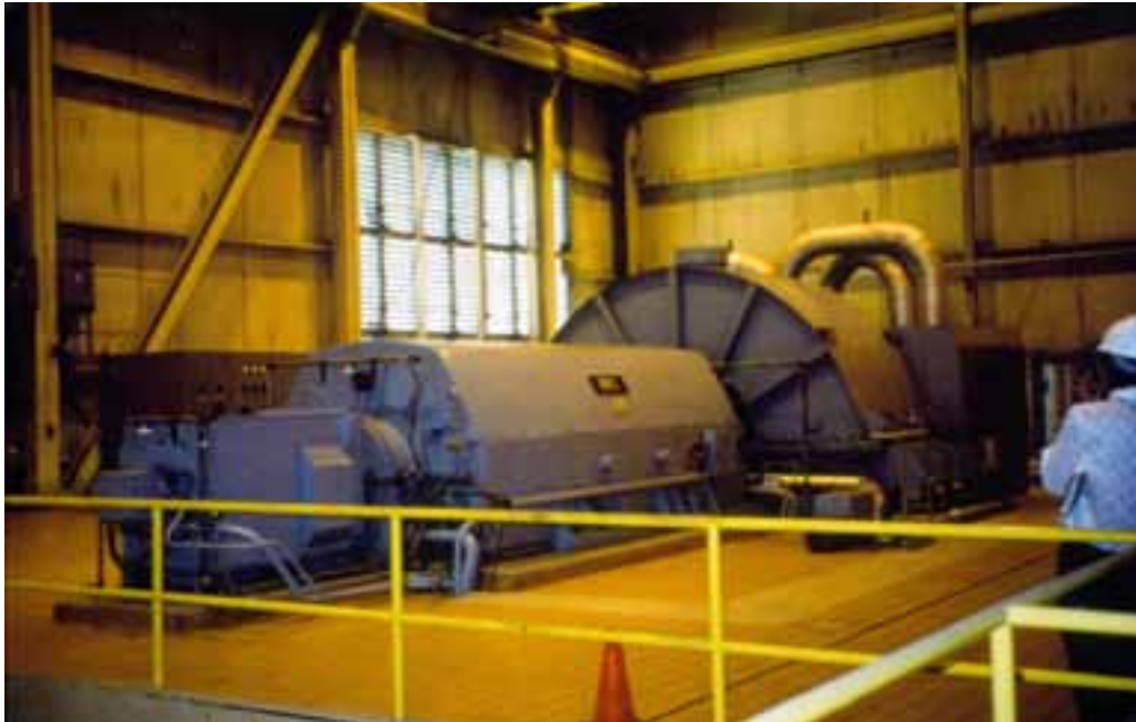
Figure 7-3: Steam turbine driving a 25 MW e generator in a wood-fired power plant in Canada
