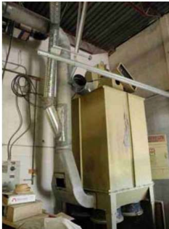
Dust collector in a mill workshop after a fire.
