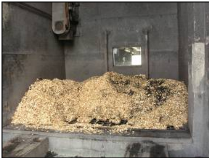
Wood chip blend at coal reception.
