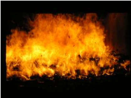
Wood chip blend grate, high fire.
