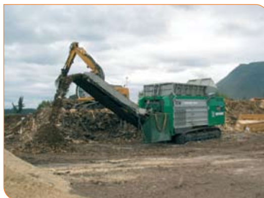
The Crambo 6000 processing wood waste into boiler fuel.
