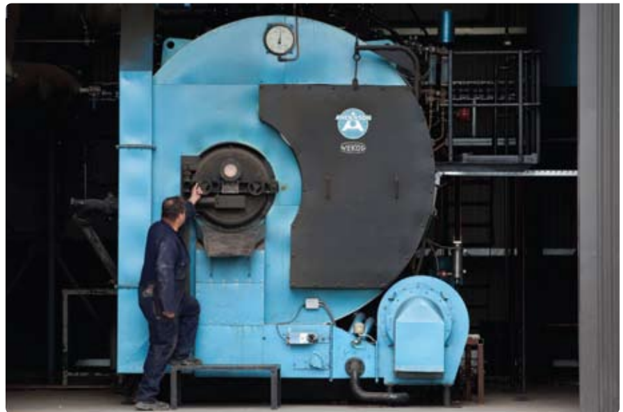
An employee checks the boiler.
